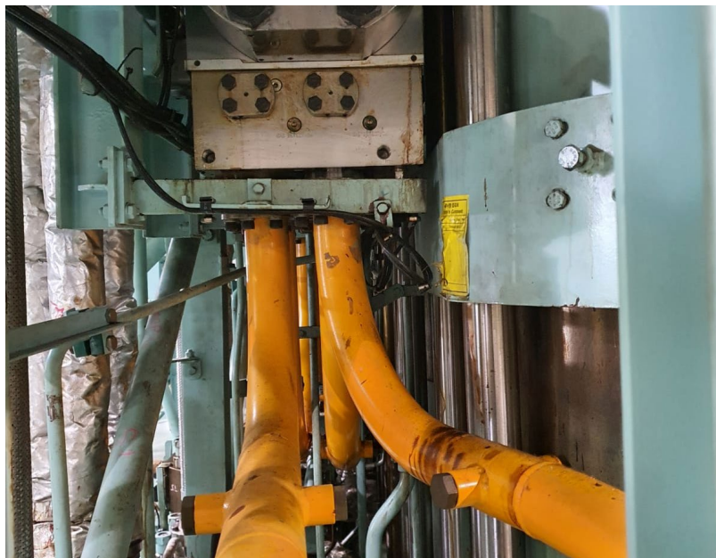
Figure 3 Fuel gas pipes
